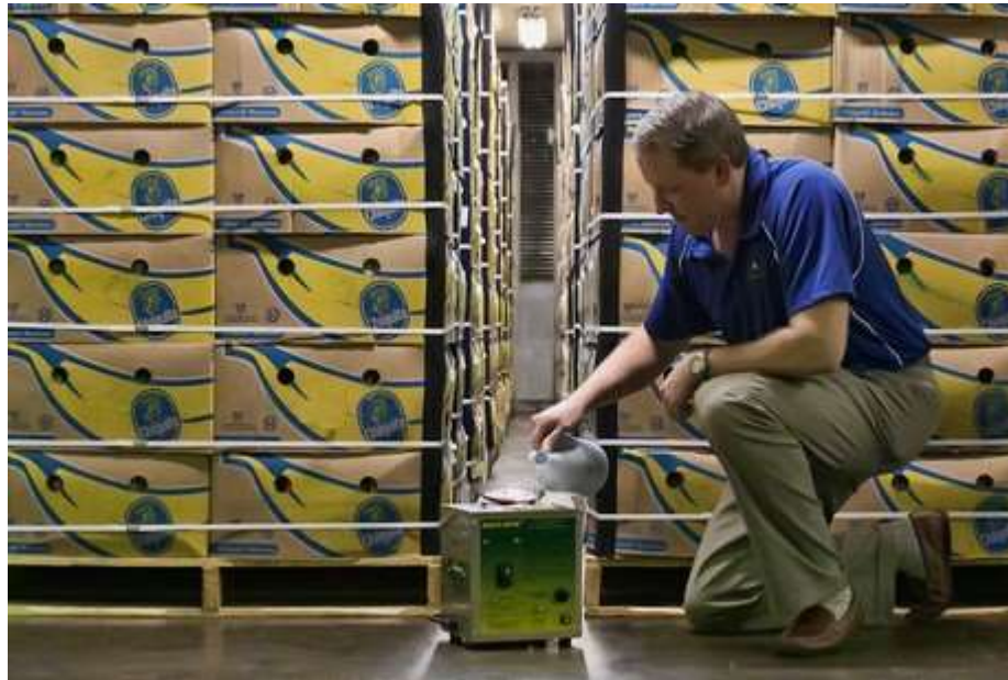
Catalytic generator for ethylene production in ripening room
